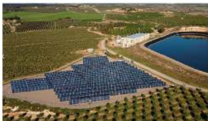
Bombament solar 500 Kwp Bombeo solar
